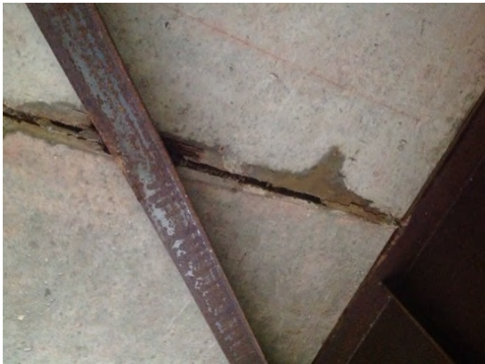
water getting through 1 deck joint
